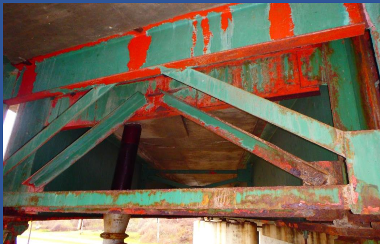
End diaphragm at Pier 3 with peeling paint and laminated rust.
