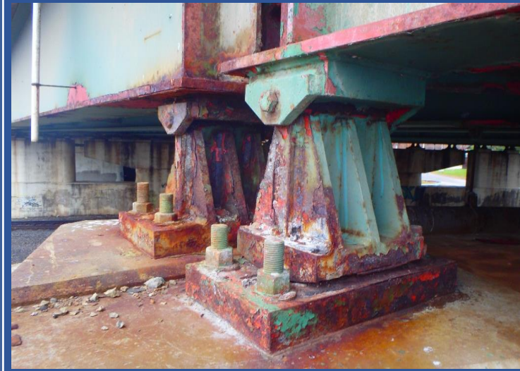
Expansion Rocker Bearing with 1/8" thick pack rust under rocks and Fixed Bearing with moderate rust and peeling paint at Pier 3.
