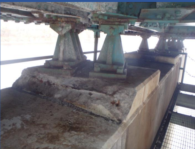
Spall at pedestal with exposed rebar (Pier 7).
