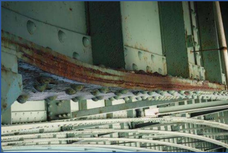
Pack rust between plates at the bottom flange.
