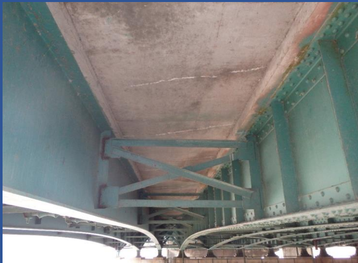
Condition of underside of deck (Span P10).
