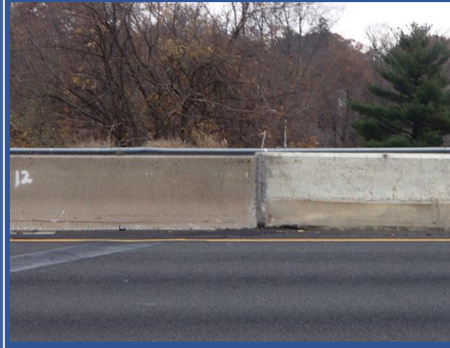
Approach median barrier at Abutment No. 1, settled approach median.
