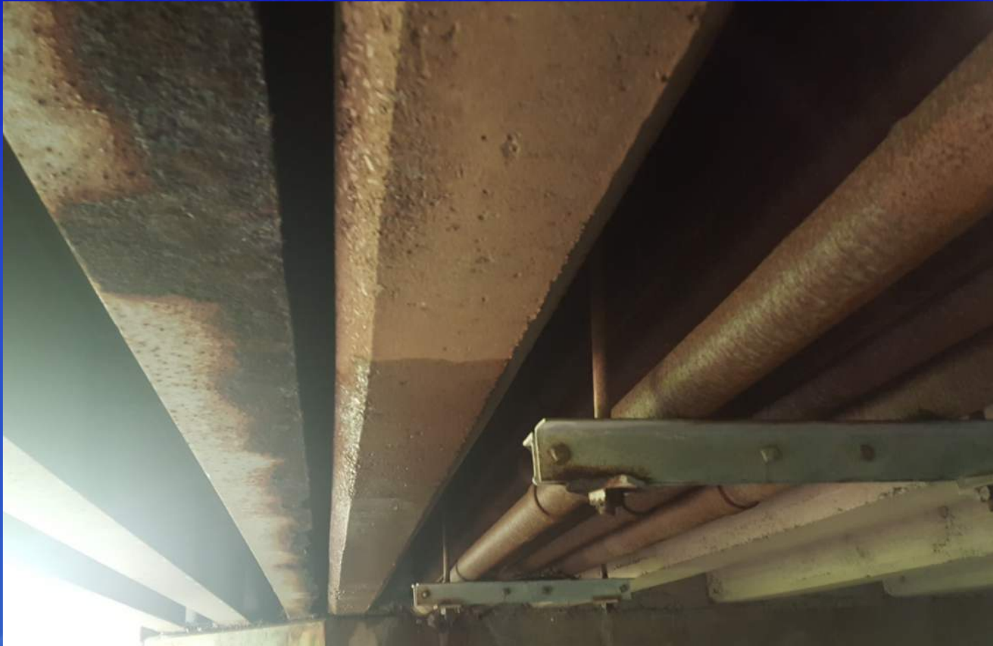
Frontier Conduits below Bridge (Looking West)
