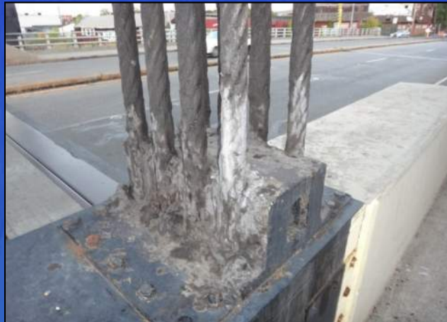
Counterweight Rope Connection External View
