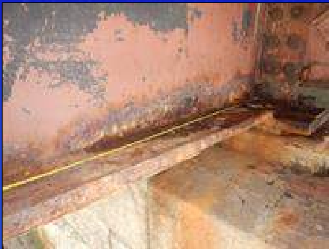
Deterioration to steel, Girder 9, Span 6 shown
