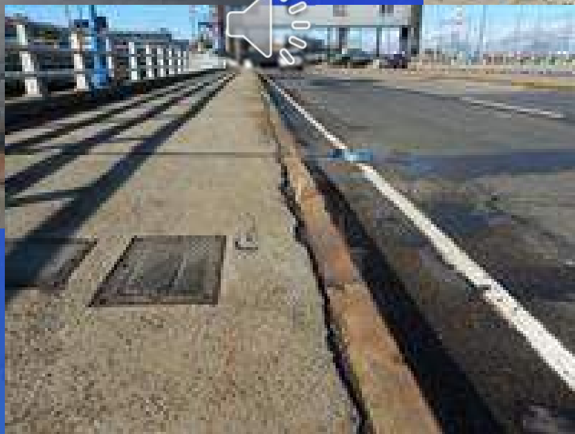
Cracking and deterioration to concrete along south sidewalk
